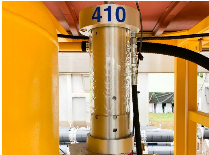
In-line gas and water content measurement
